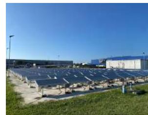
For Nestlé (BR) process heat for a dairy factory
