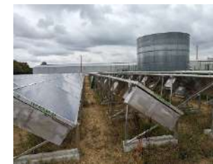
For Larnaudie (FR) boiler fw preheating for food factory
