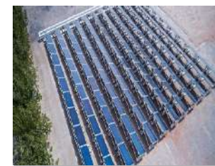
For ORF (UAE) process heat for a rubber factory
