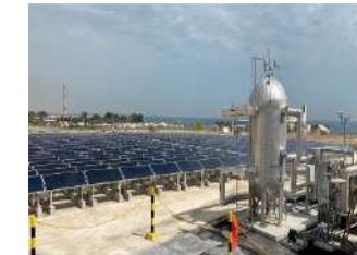
For Aramco (KSA) boiler fw preheating for an oil facility
